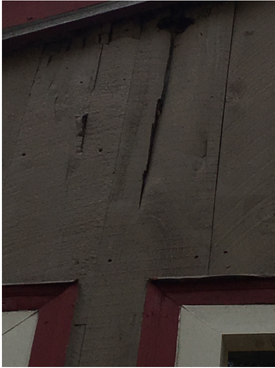
Figure 3. East Wall - Rain & Humidity Damage.
