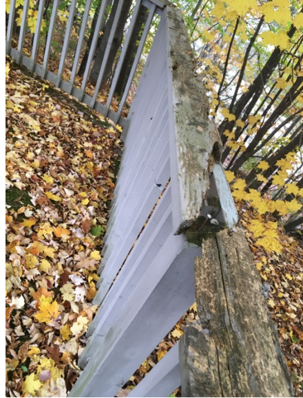
Figure 13. Rotted Fence Sections.
